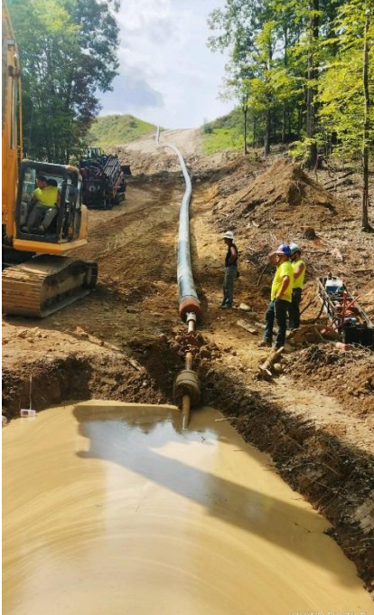
Workers prepare to pull 400' of 16" x 12" HDPE water main below RT93 in September 2018.
