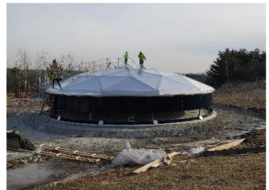
December 2018 – After months of preparation, the new 1MG glass-fused-to-steel water storage tank begins to take shape. Phase 1 completion is scheduled for June 2019 at a cost >$2M.
